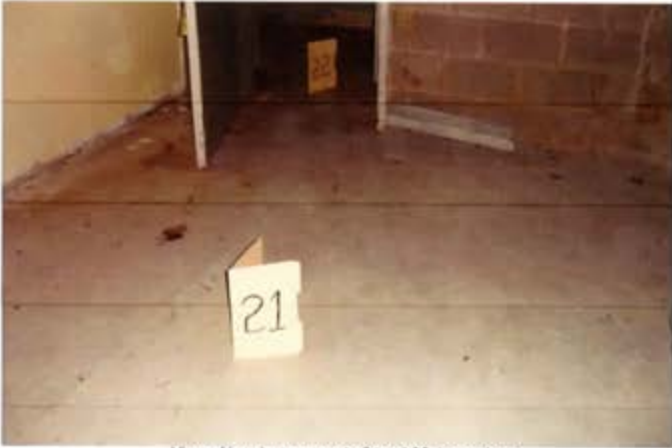
View of Lead wipe sample 21 and 22, located on the floor 6 feet from the exit door and outside the in hallway
