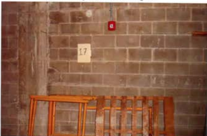
View of Lead wipe sample 17, located on right wall in the IFR Posted to NGB FOIA Reading Room May, 2018
