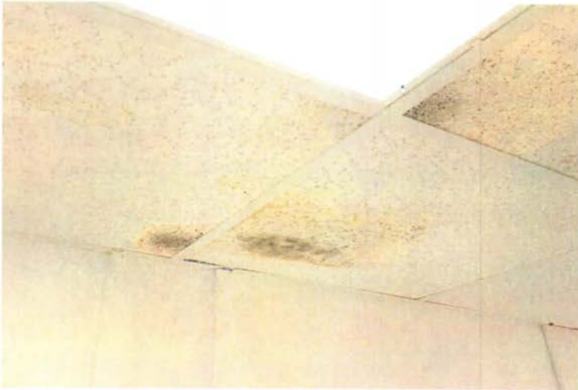
Photo #3: Water stained ceiling tiles in the distance learning center.
