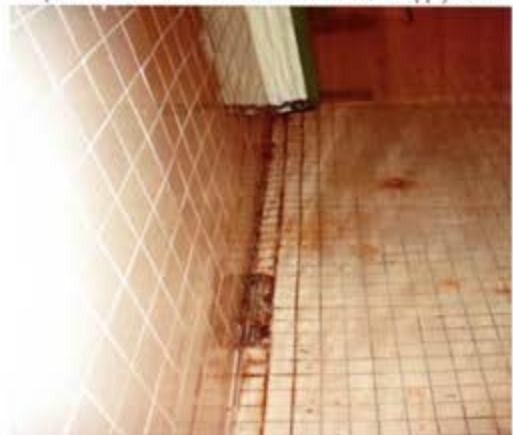
View of possible moisture damaged floor tiles in the kitchen FOIA Requested Record #J-15-0085 (VI) Released by National Guard Bureau Page 178 of 389
