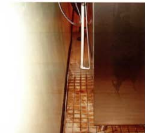
View of floor where water is leaking from ice machine in the kitchen Posted to NGB FOIA Reading Room May, 2018
