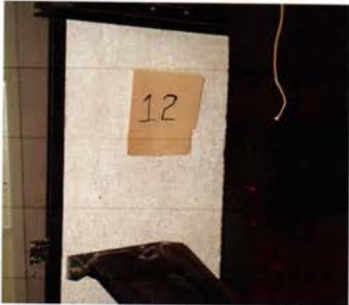
View of Lead wipe sample 12, located on acoustic wall at firing line 3
