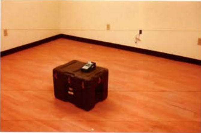
View of mold sampling within room that had previous mold issues
