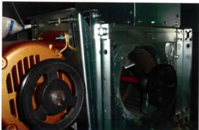
View of the fan assembly located within the AHU that is missing a fan belt
