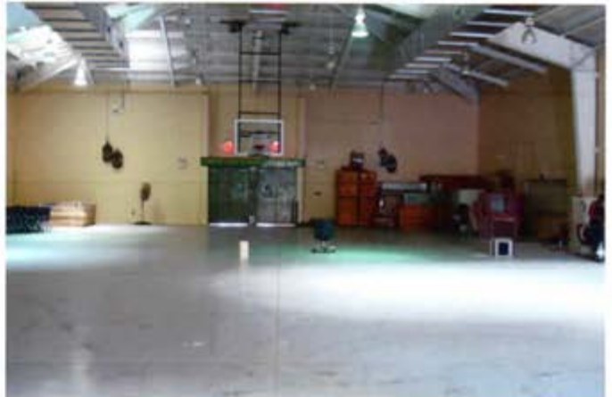
View of the Drill Hall and Lead wipe sample 2, located on the center of drill hall floor
