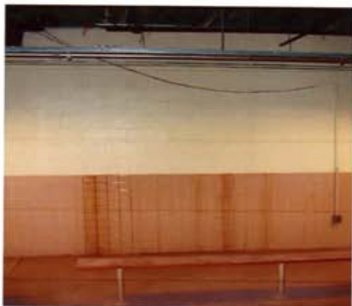
View of water stained wall located in the former locker room
