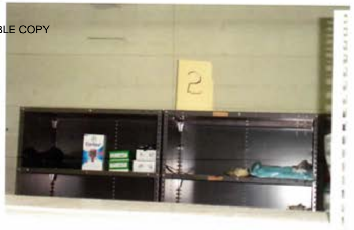
View of Lead wipe sample 2, located on the shelf in the Medical company supply room
