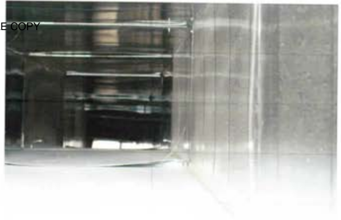
View inside closed duct from AHU 5 leading into Indoor Firing range. AHU is not in service.
