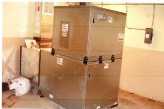
View of AHU 8, located in the former locker room. The AHU is not in operation
