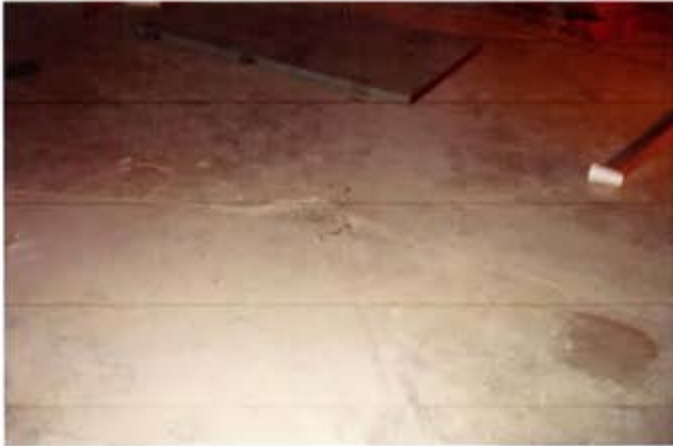
View of the sinking and cracked floor in the IFR
