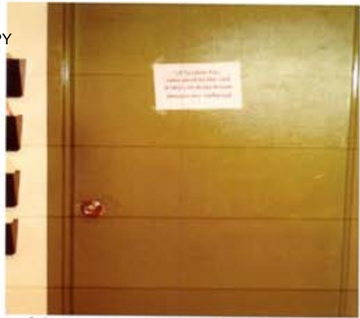
View of door to area that had previous mold issues
