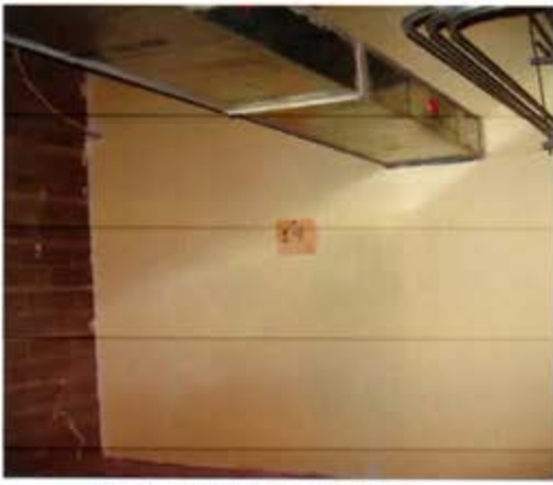
View of Lead wipe sample 19, located on the rear wall right side in the IFR
