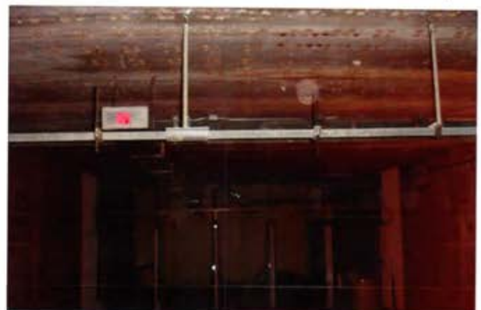
View of concrete ceiling of the indoor firing range. Acoustic material and light buffers removed
