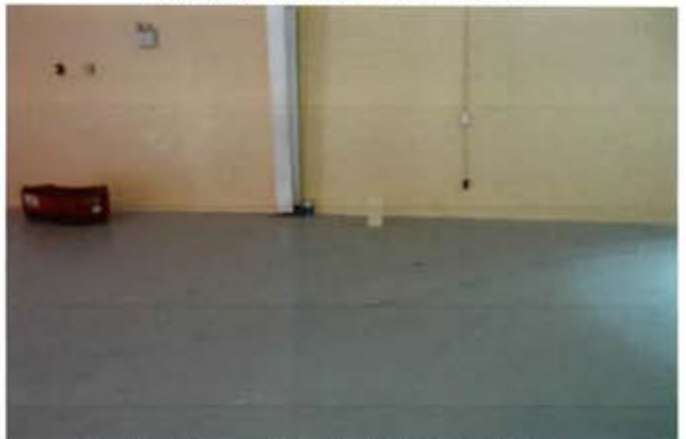
View of Lead wipe sample 4, located on the right side of the Drill hall
