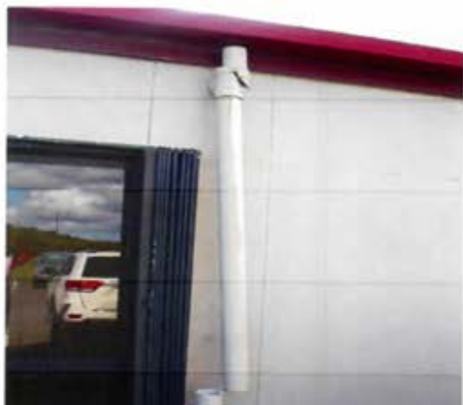
View of cracked downspout
