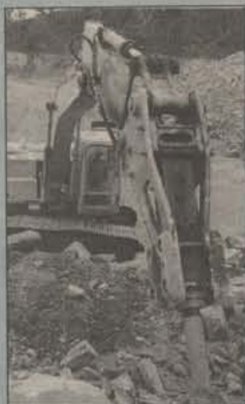
PAVING THE WAY - Missouri's Lt. Col. King Sidwell (center) peers through a culvert. An Army Guard engineer (left) puts some heavy equipment to work. Navajo President Albert Hale (below, left) greets a Guardmember.
