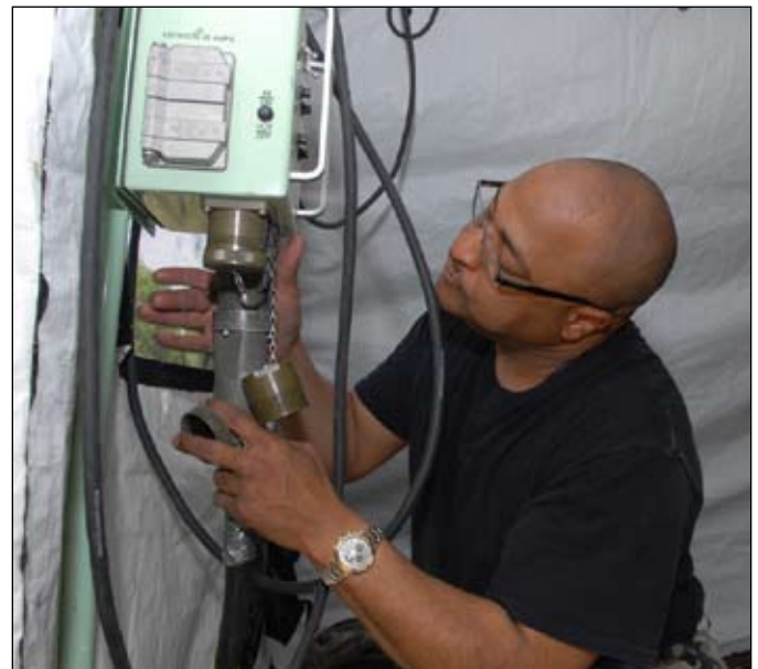
Tech. Sgt. David Betts, of the 187th Medical Group, assembles an electrical distribution panel in a field hospital in preparation for the Vigilant Guard 2008 exercise on April 19, in Beaufort, S.C. (DoD photo by Senior Master Sgt. David H. Lipp) (RELEASED)
