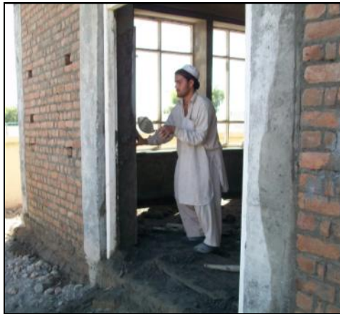
A worker tuck points brickwork at the Rodat Agriculture Extension Center. Future construction of agriculture extension centers will be approved through the CERP as a Budget process.
