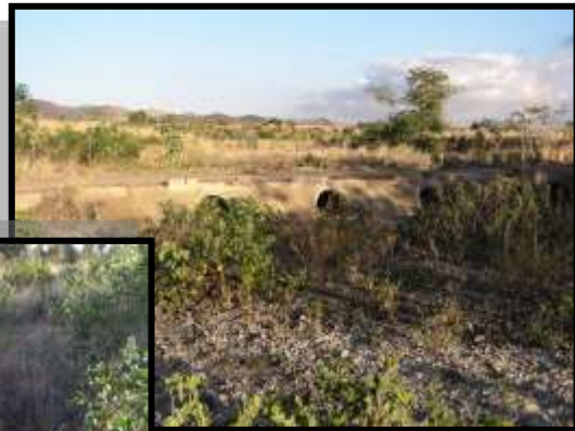
Blue Route Point 13 - Plugged
