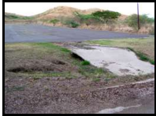
Drainage erosion off parking lot at Point 3 along the Blue Route.
