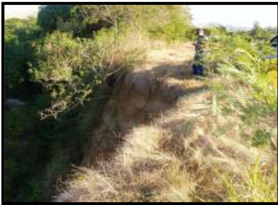
Quebrada Honda bank erosion at Point 17
