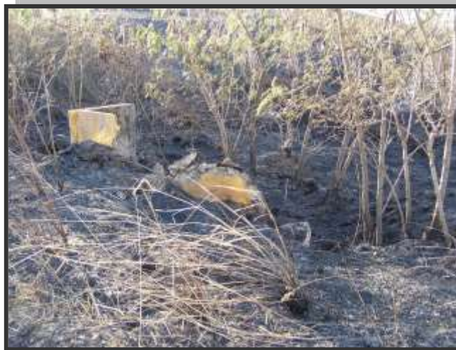
Damaged inlet structure at Point 12 along the Blue Convoy Route.
