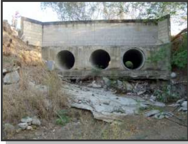
Outlet of the 60-inch triple barrel crossing at Red Convoy Route Point 14.
