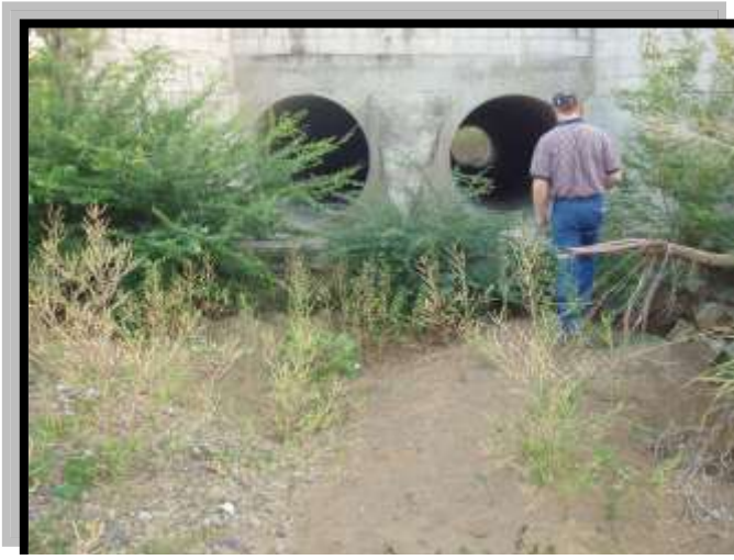
Outlet of the 60-inch double barrel crossing at Red Convoy Route Point 13.
