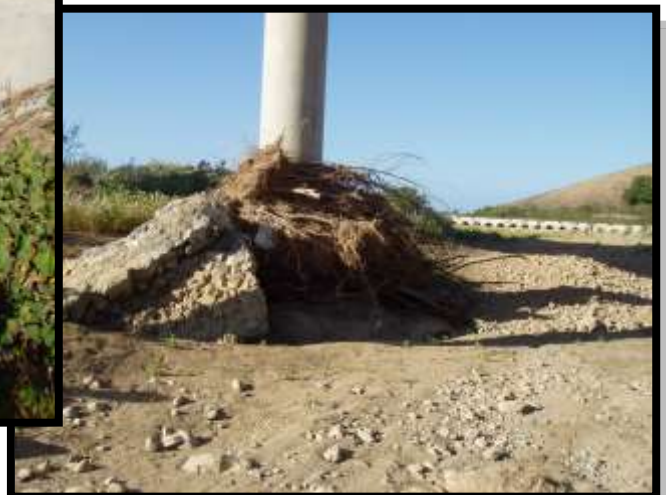
Scour/erosion around main entrance bridge columns
