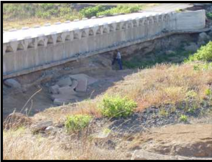
Downstream view and toe scour along the lower entrance crossing.
