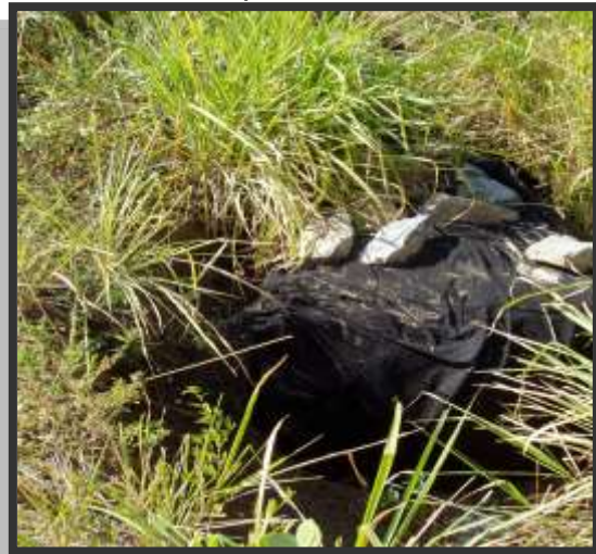
Erosion around gabion, Orange Route Point 4
